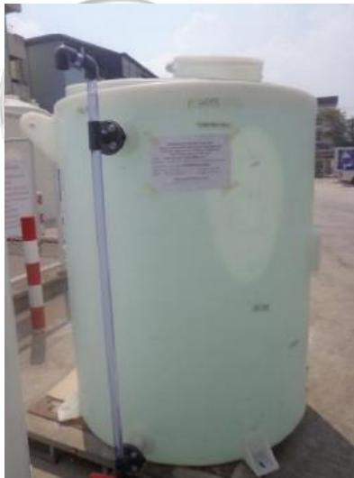
Urea Tank - 2m 3
