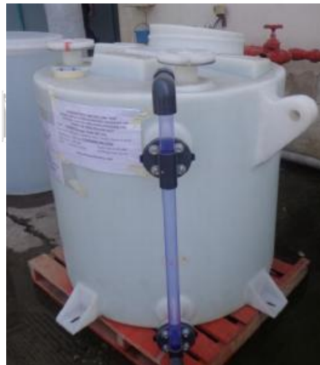
H 3 PO 4 Tank - 0.5m 3
