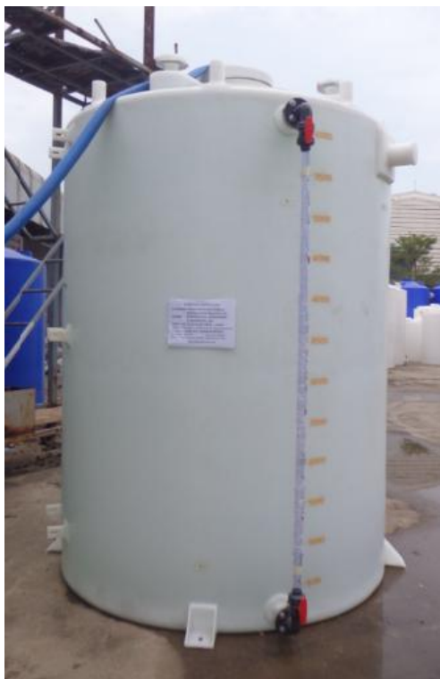
NaOH Tank - 6m3
