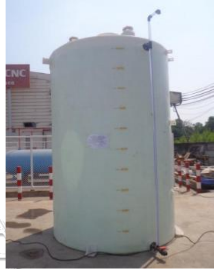
NaOH Tank - 10m 3
